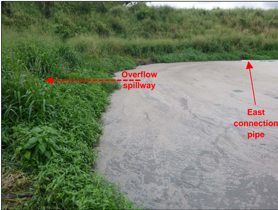
Photograph 31. View, facing south, of the approximate location of the lower lagoon overflow spillway. Photo by A. D'Angelo; 12/14/16.
