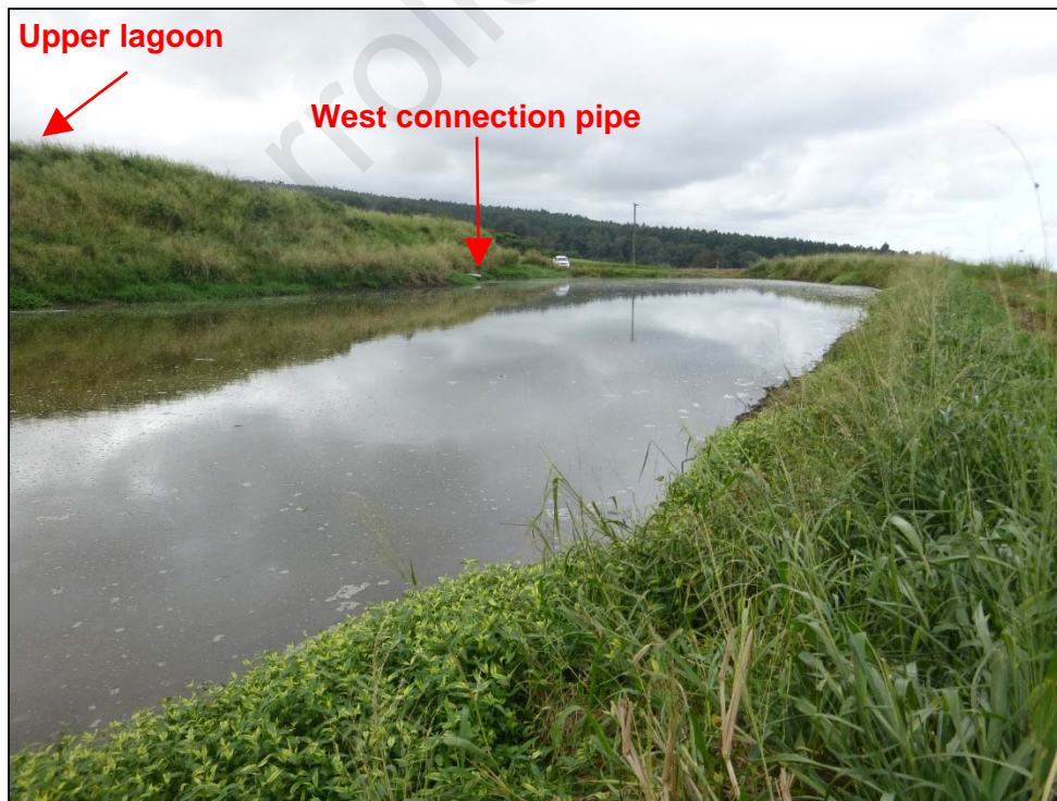
Photograph 26. View, facing west, of the lower lagoon. The lagoon was near capacity at the time of the inspection and was not equipped with a depth marker. Photo by A. D'Angelo; 12/14/16.
