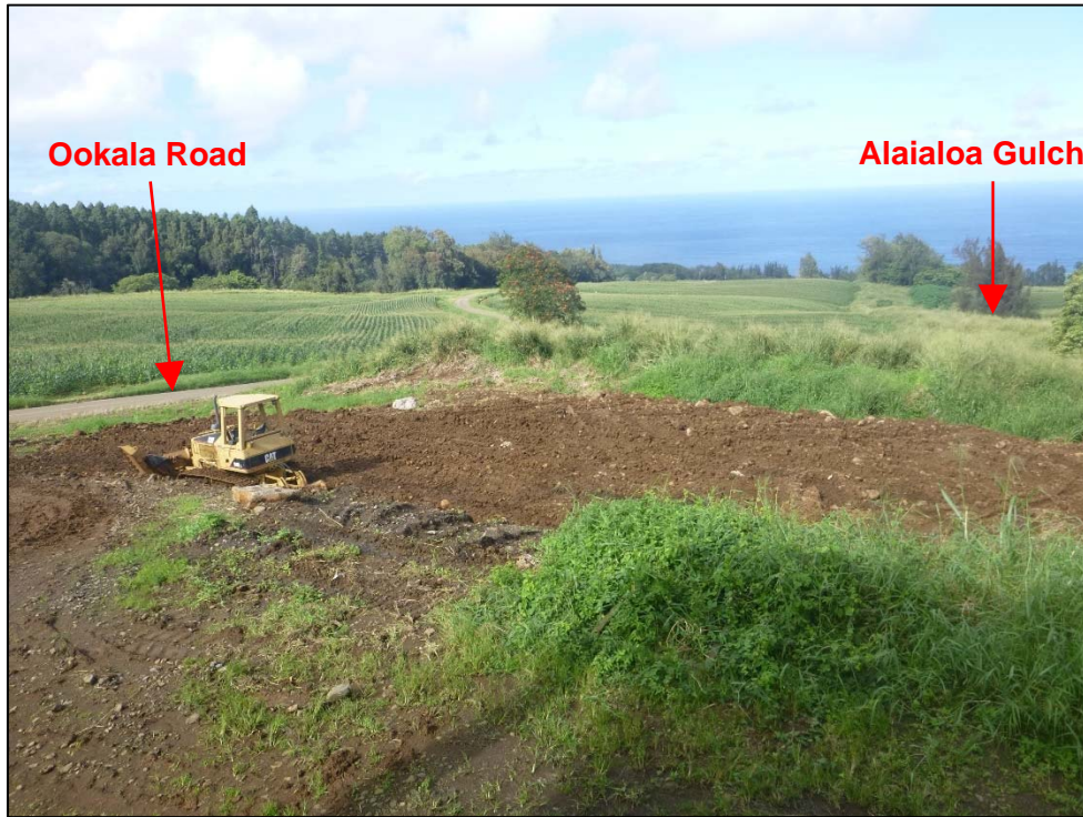
Photograph 21. View, facing north, of a disturbed area near Ookala Road. This area will be paved to store the honeywagon shown in Photographs 15 and 20. I observed a vegetated buffer between the disturbance and Alaiialoa Gulch. Photo by A. D'Angelo; 12/14/16.
