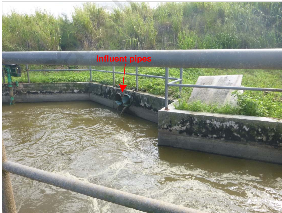
Photograph 16. View of the manure composting building collection pit influent pipes. Photo by A. D'Angelo; 12/14/16.
