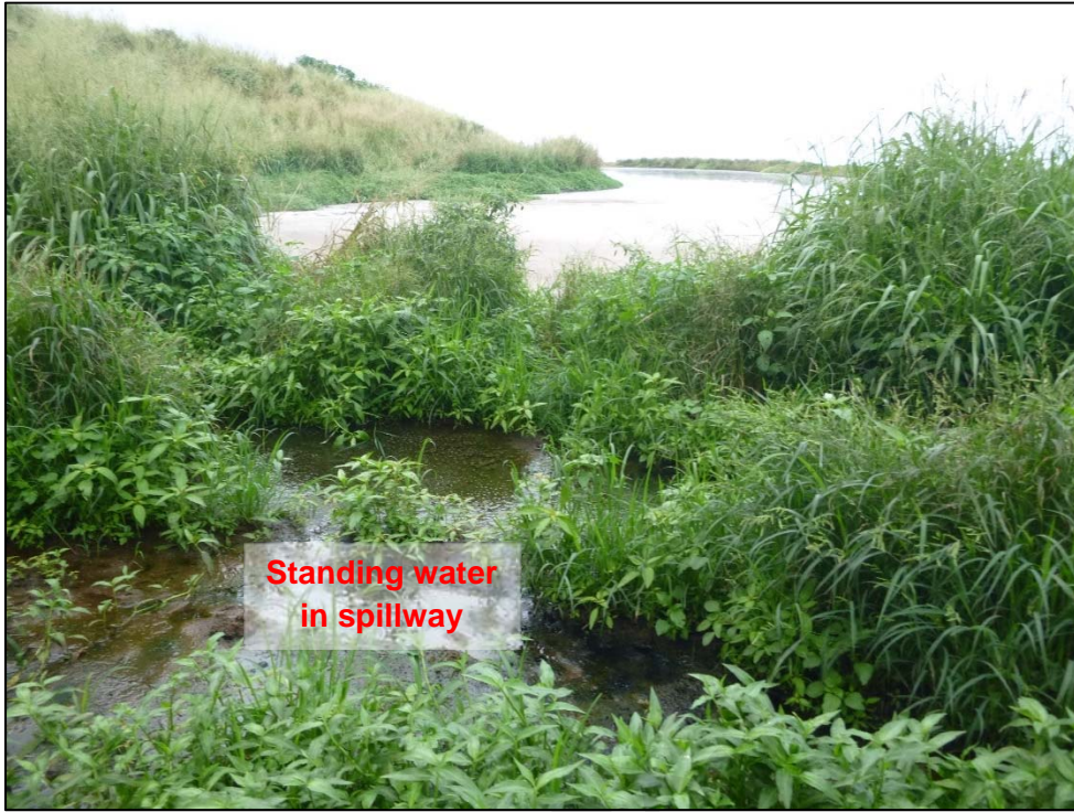
Photograph 33. View of algae growth and standing water in the lower lagoon overflow spillway. Photo by A. D'Angelo; 12/14/16.
