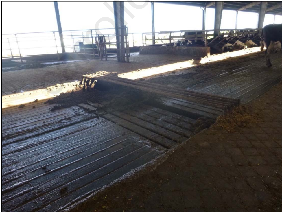
Photograph 8. View of the manure collection trough in the center of the lower freestall barn. The contents of the collection trough gravity flow into a collection pit located at the manure composting building, shown in Photographs 15 and 16. Photo by A. D'Angelo; 12/14/16.
