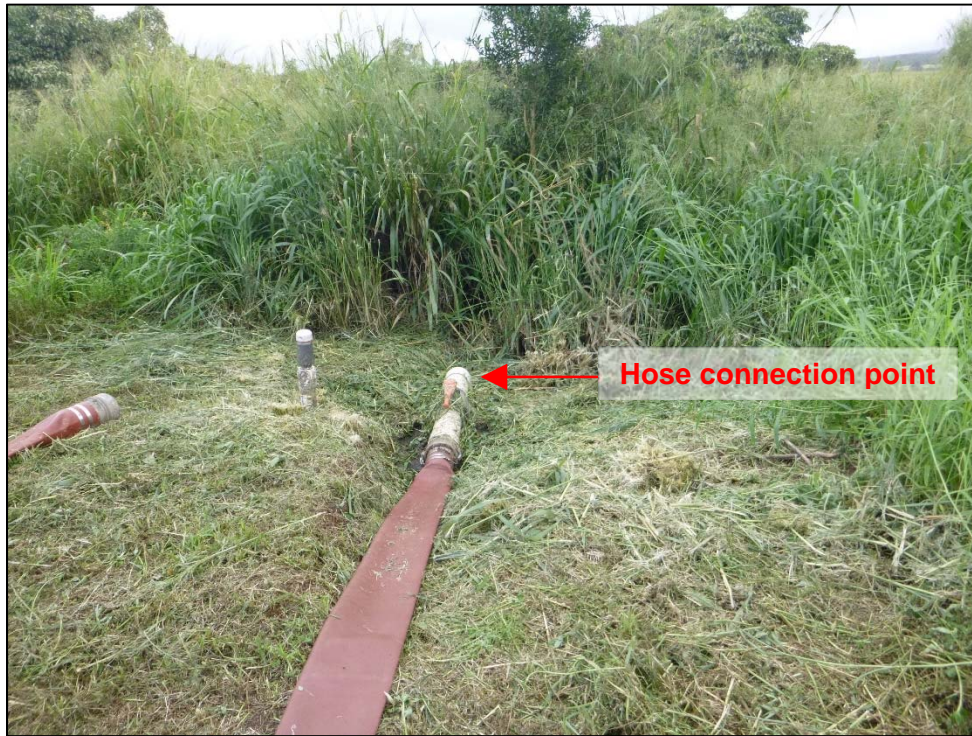
Photograph 29. View of the draw pumping system hose connection point to the Facility's irrigation system. Photo by A. D'Angelo; 12/14/16.
