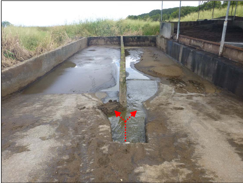
Photograph 23. View of flow from the manure composting collection pit entering the primary cells of the manure solids separation cells shown in Photograph 22. Photo by A. D'Angelo; 12/14/16.
