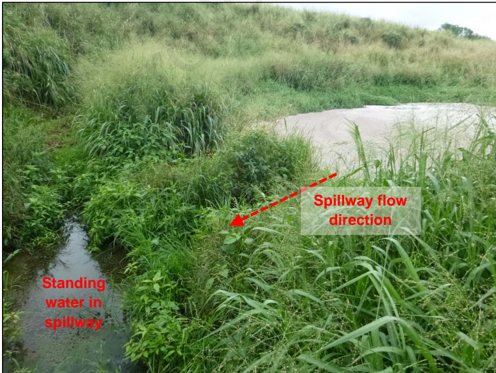
Photograph 32. View, facing southwest, of the lower lagoon overflow spillway. Note the presence of algae growth and standing water in the overflow spillway. Photo by A. D'Angelo; 12/14/16.
